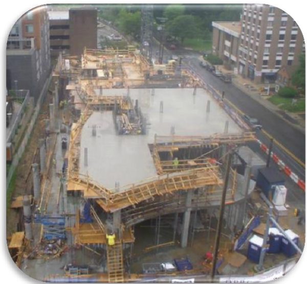
Figure 3.2 - Aerial construction camera looking at the third floor construction: Courtesy of United Therapeutics and Oxblue.com
