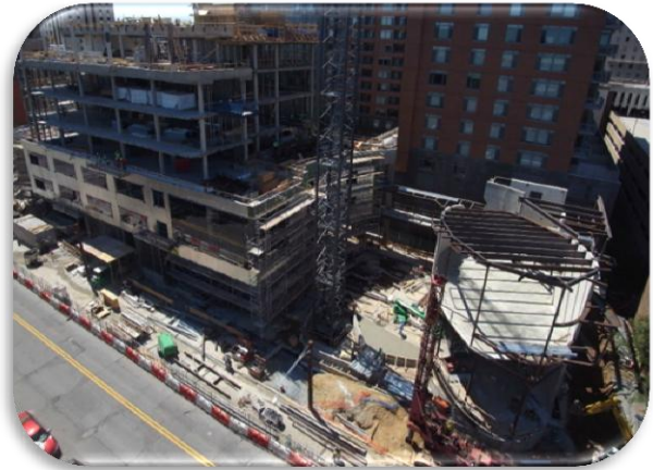
Figure 3.1- Aerial construction camera looking at the Unitherium roof framing: Courtesy of United Therapeutics and Oxblue.com
